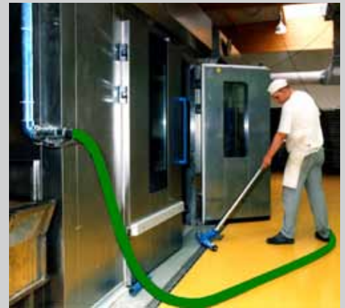
Vacuum cleaning of an oven unit with a stationary vacuum system
