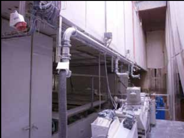
Cleaning of production machinery. Vacuum cleaning of production equipment
