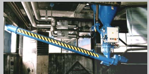
Stationary vacuum cleaning unit with pipework system
